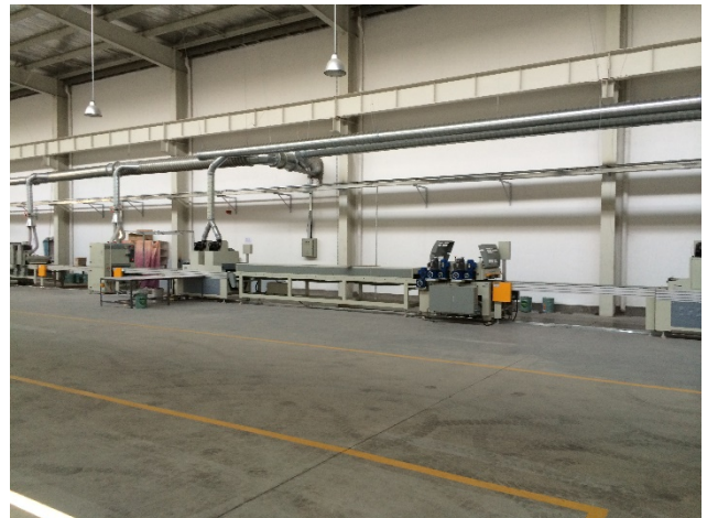
Finishing Line 9 application stations
